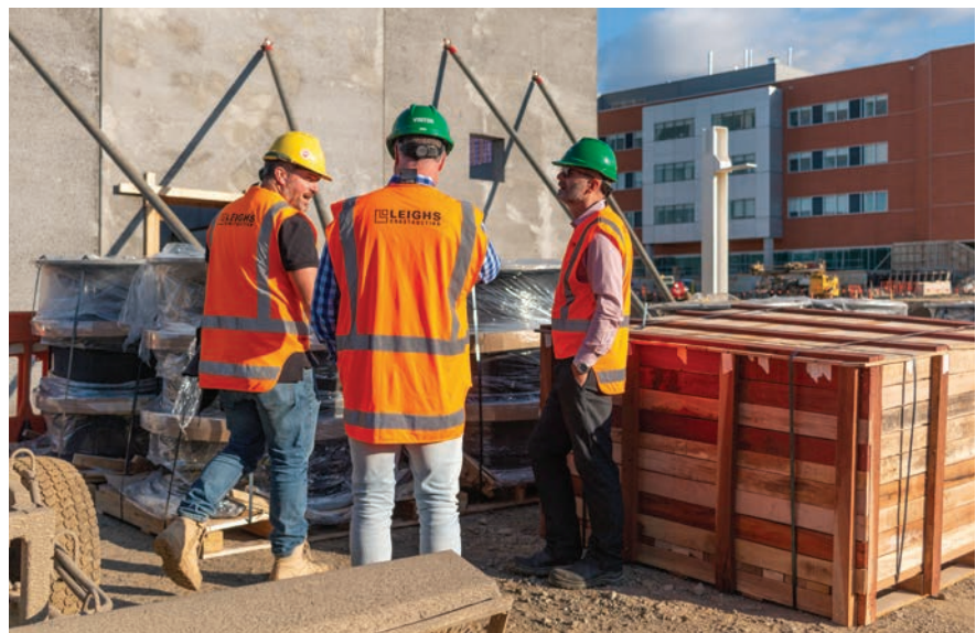
Leighs project manager Nathan Hawkins shows Adrian Sole and Grant Carter some of the base isolators on the Project Maunga site.
